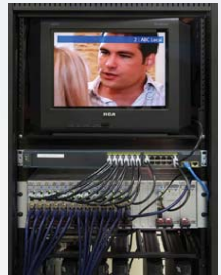
VSI Media Processing Platform at Metro (the system includes four platforms with 57 AVN-220 encoder blades installed)
